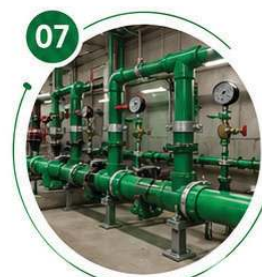
07 Heating system main lines.
