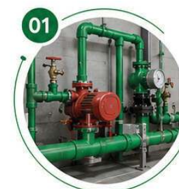
01 Hot water distribution systems.
