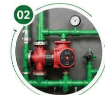
Hot water circulation systems
