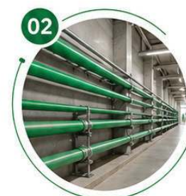
02 Long pipe runs requiring minimal expansion.
