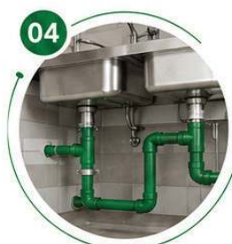
04 Commercial plumbing systems.
