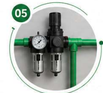
Compressed air systems
