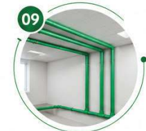
Radiant heating and cooling
