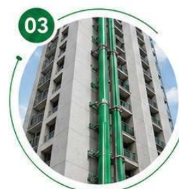
03 High-rise building installations.
